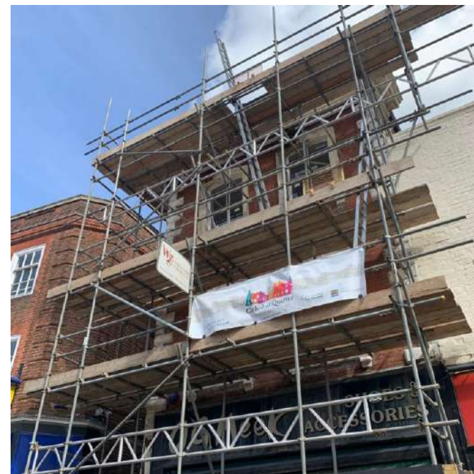
Works at 14 Westgate Street as part of the Cathedral Quarter HSHAZ. Photo: GCC.
